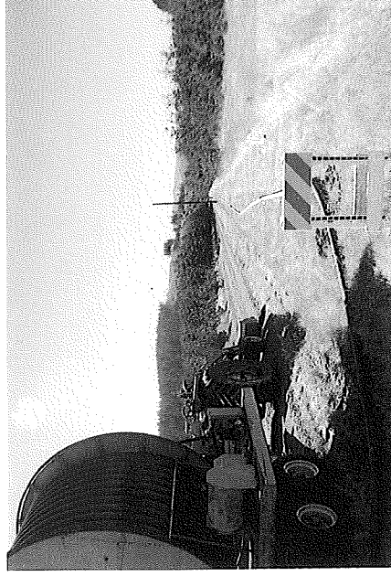
Figure 4 Reel line to field
