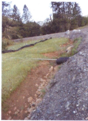
Using culvert to route sprinkler pipe to irrigate middle of WR May 6, 2014 at 7:30:07 AM
