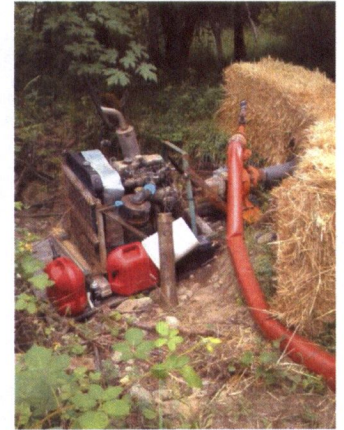
Pump used at POD for sprinklers June 12, 2013 at 10:46:13 AM
