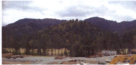
Looking down from corner of property towards SE corner of WR June 12, 2013 at 9:48:42 AM
