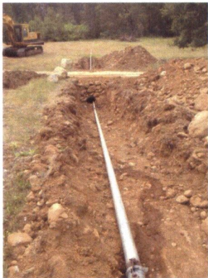
Pipe installed near POD under road to feed irrigation system June 12, 2013 at 10:47:28 AM
