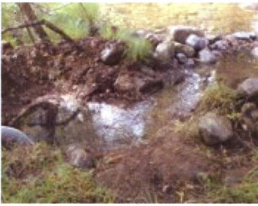
Pump sump at diversion June 7, 2013 at 8:35:10 AM
