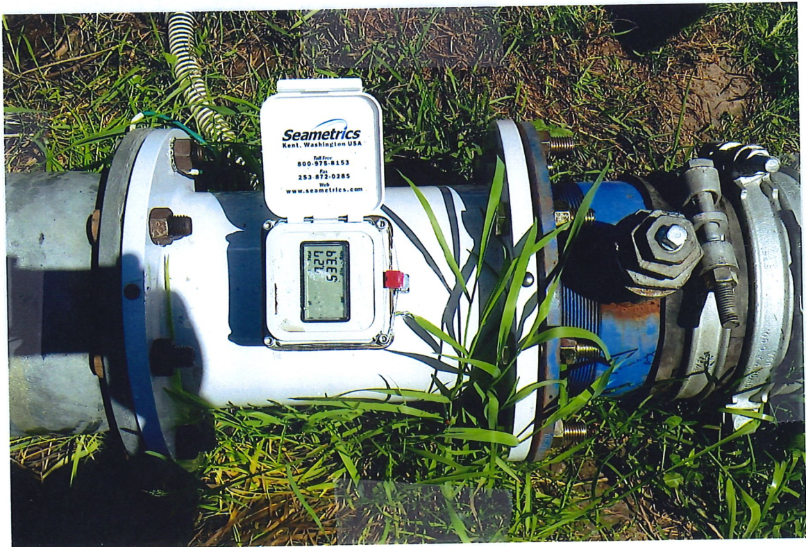
NEW FLOW METER
