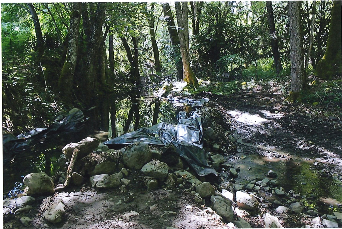
Figure 1: Push Up dam diversion structure installed in Galls Creek in 2018 irrigation season looking South. ~3 ft tall ~40 ft long.
