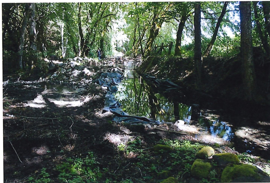
Figure 2: Push up Dam installed in Galls Creek looking downstream (North) at ditch and screens
