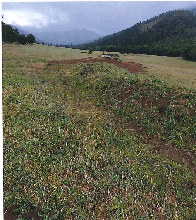
Figure 4: Existing earth irrigation conveyance ditch near beginning of water right place of use, looking South towards POD. Photo shows it being removed in early 2020 in preparation for pipeline installation and sprinkler irrigation.
