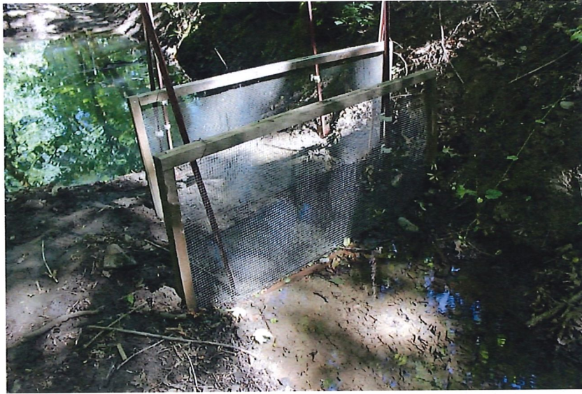
Figure 3: Fish Screens installed at beginning of ditch looking North
