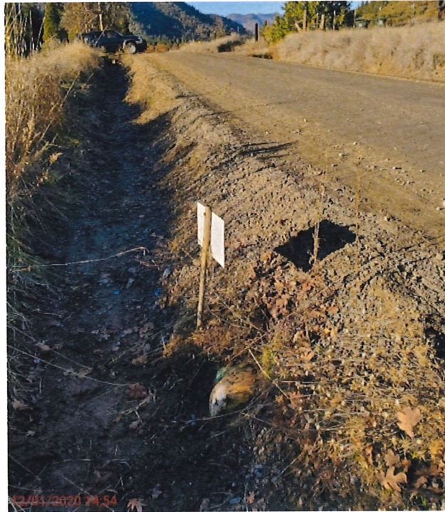
Figure 5: 10" diameter PVC piped ditch section (~300ft) under road, looking North. Water can be diverted from roadside ditch into pipe or can continue North down roadside ditch to irrigate other fields. Pipe is cleared out each season and white end cap is removed. Road was recently re-graded by county and they partially buried the pipe.
