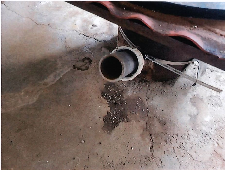
Well #3 Access Port
