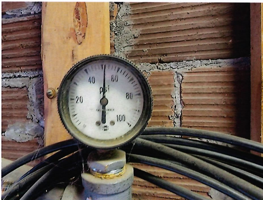
Well #2 Pressure Gauge
