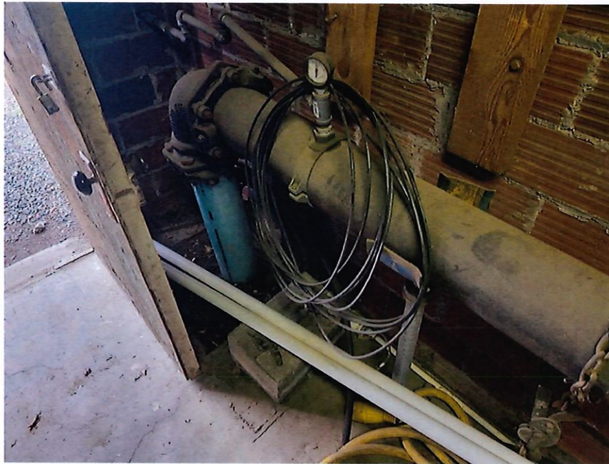
Well #2 Discharge to Municipal System
