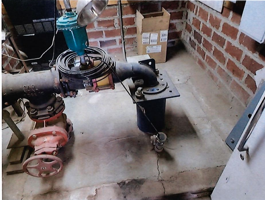
Well #2 & Access Port
