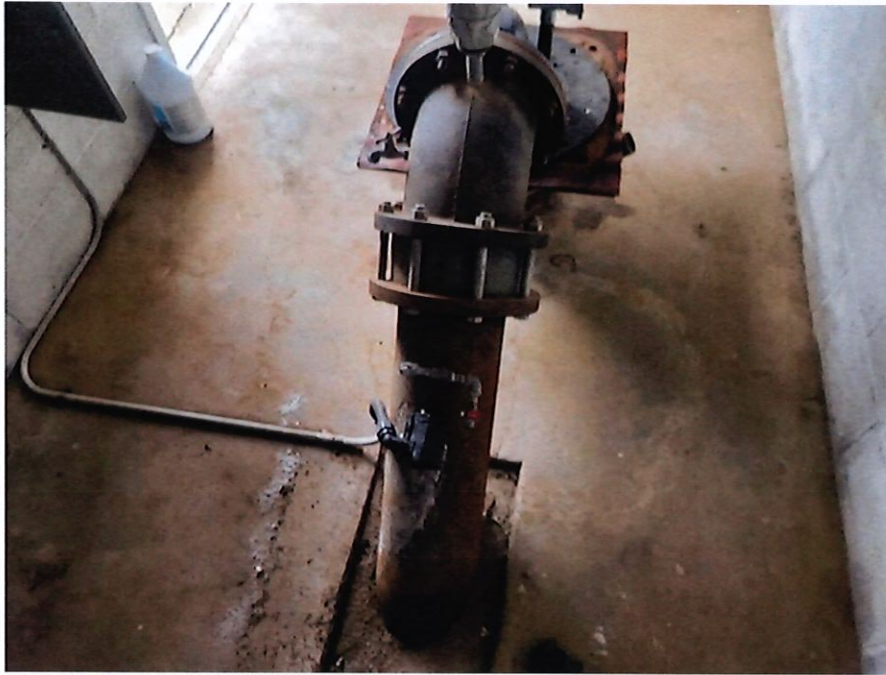
Well #3 Discharge to Municipal System
