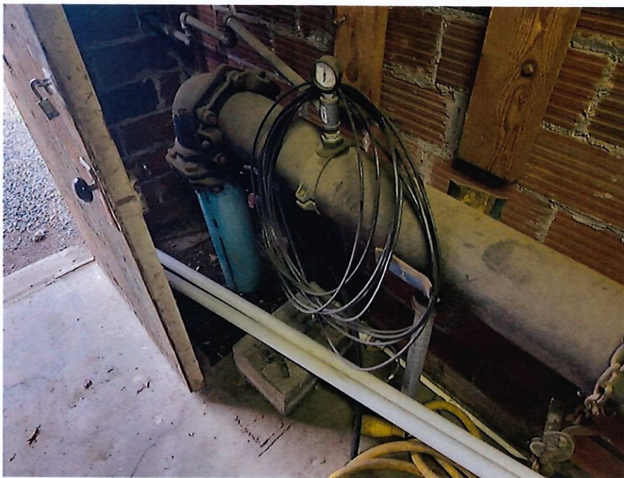
Well #2 Discharge to Municipal System
