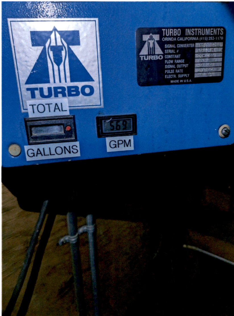
Figure 1. Flowmeter information at Willamette Pass snowmaking system
