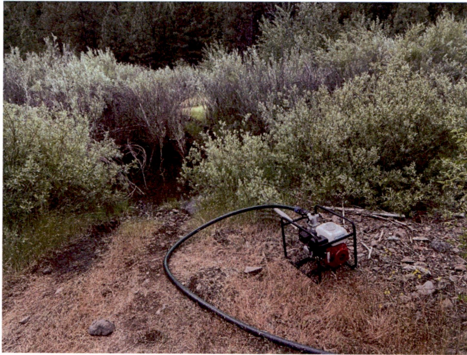
Figure 21: POD 11 with pump station in operation
