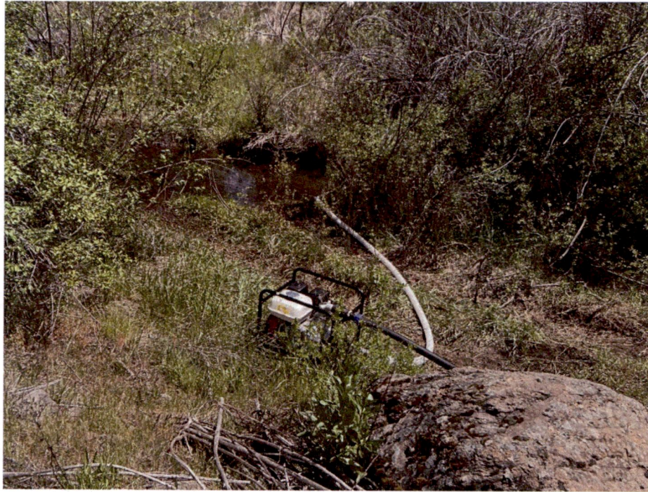
Figure 19: POD 8 with pump station in operation
