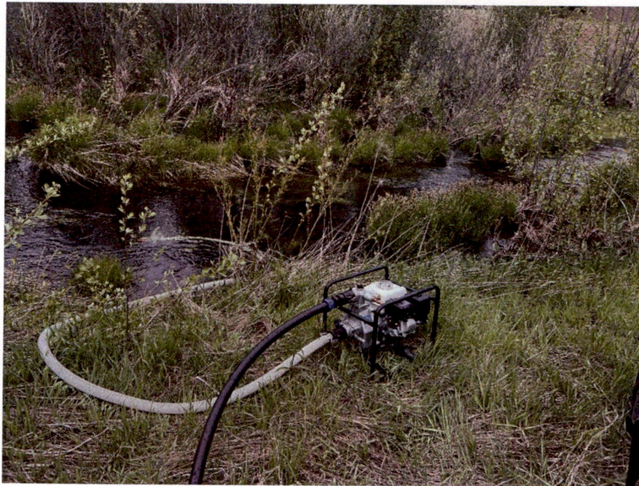
Figure 12: POD 1 with pump station in operation
