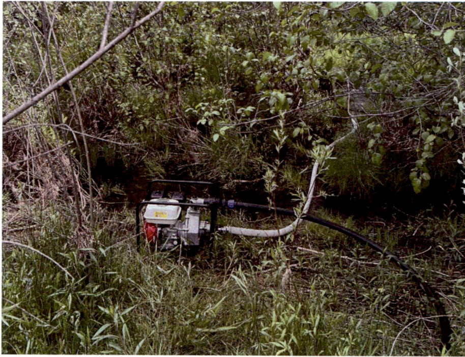
Figure 17: POD 6 with pump station in operation
