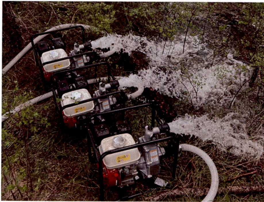
Figure 22: POD 12 with pump station in operation
