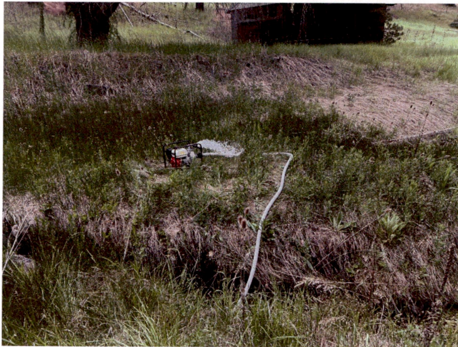
Figure 14: POD 3 with pump station in operation
