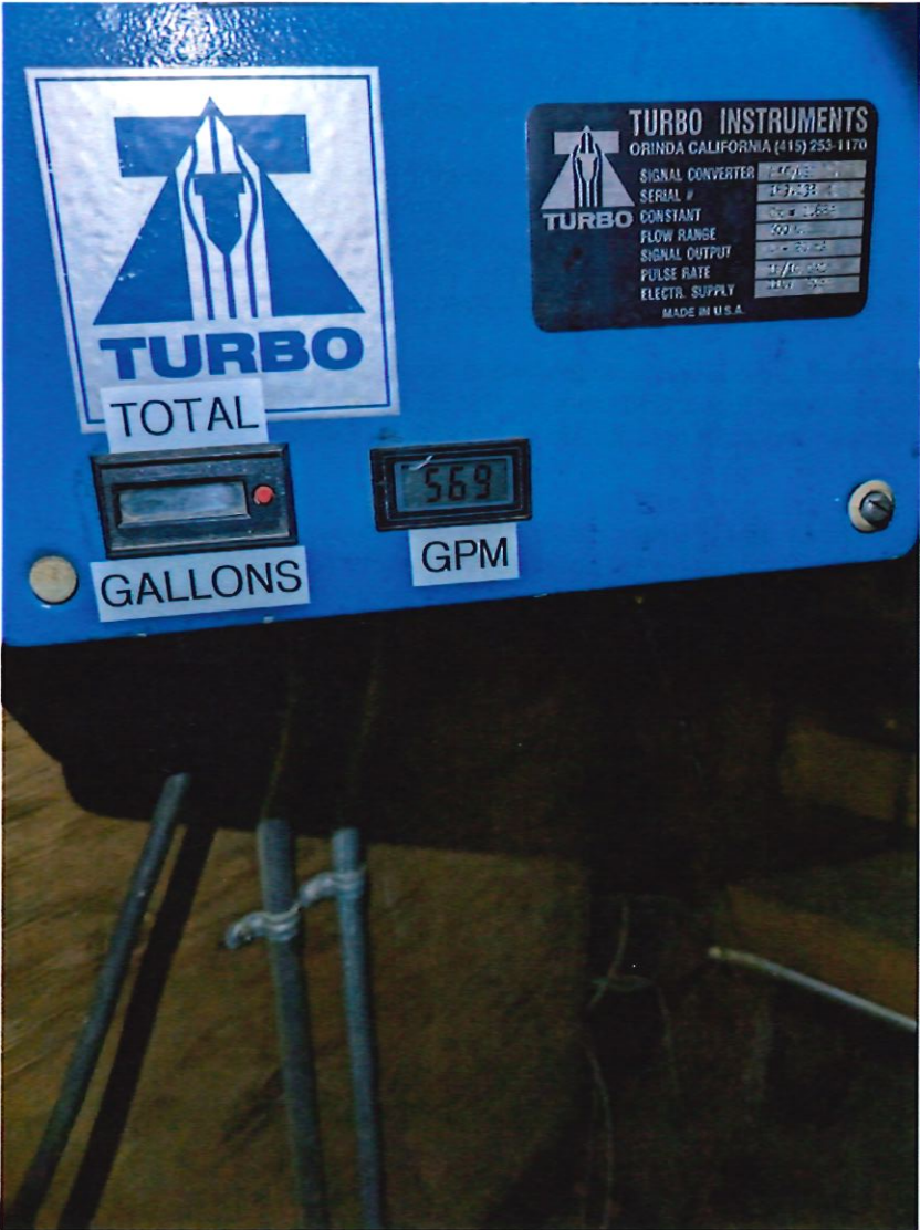
Figure 1. Flowmeter information at Willamette Pass snowmaking system
