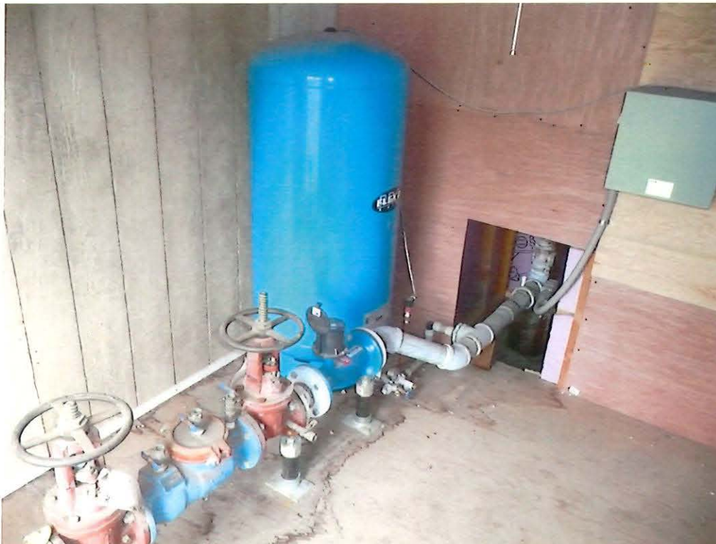
Picture of Well #4, in background in doghouse, meter is shown in front of pressure tank.
