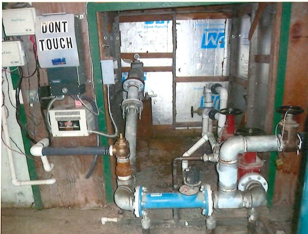
Picture inside the pump house showing Well #2 in the background, the meter in the foreground.
