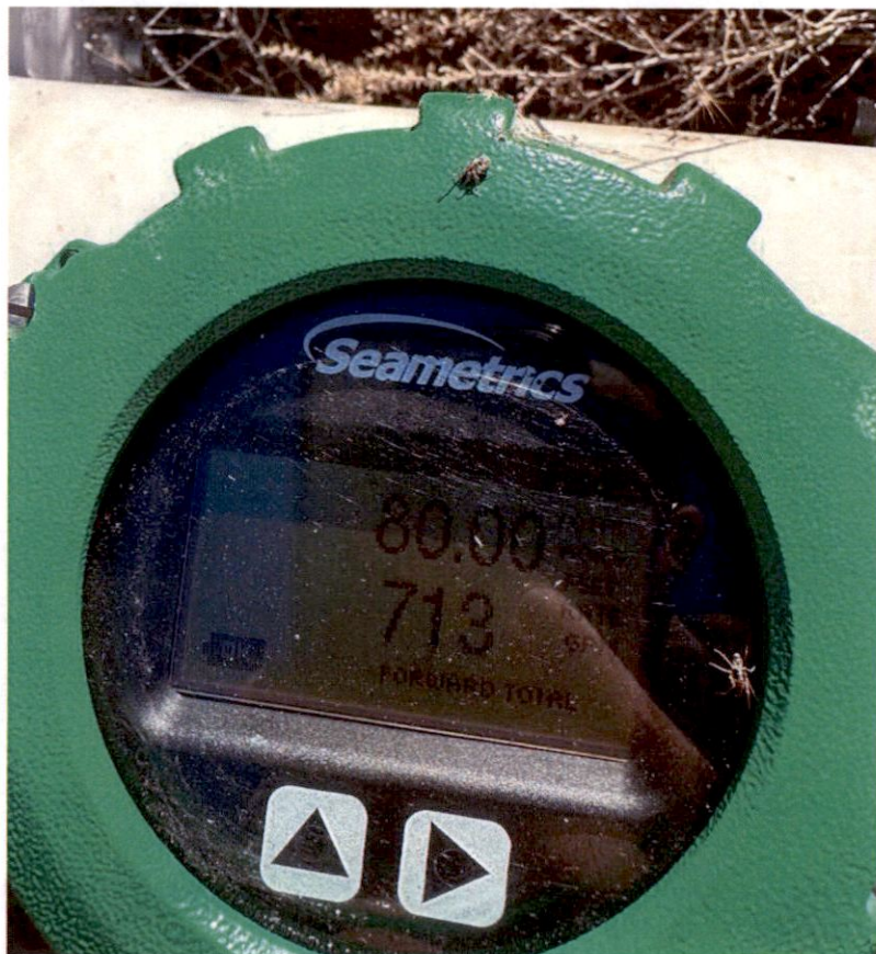
Figure 1 - Flowmeter at completion of release
