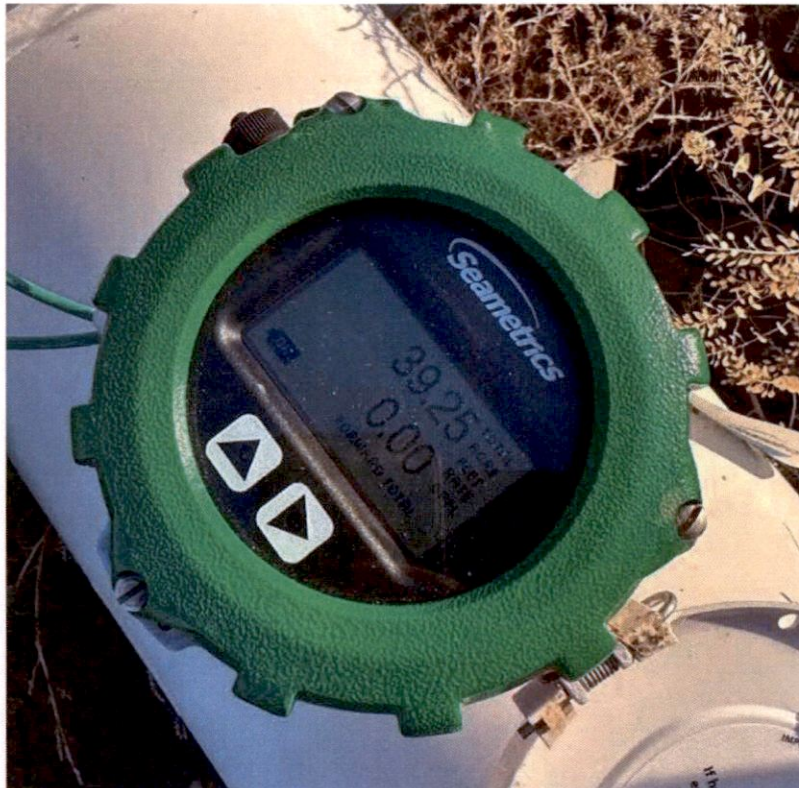
Figure 1 - Flowmeter at completion of release
