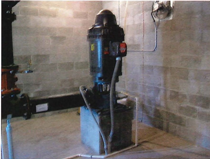
PUMP AND MOTOR ASSEMBLY
