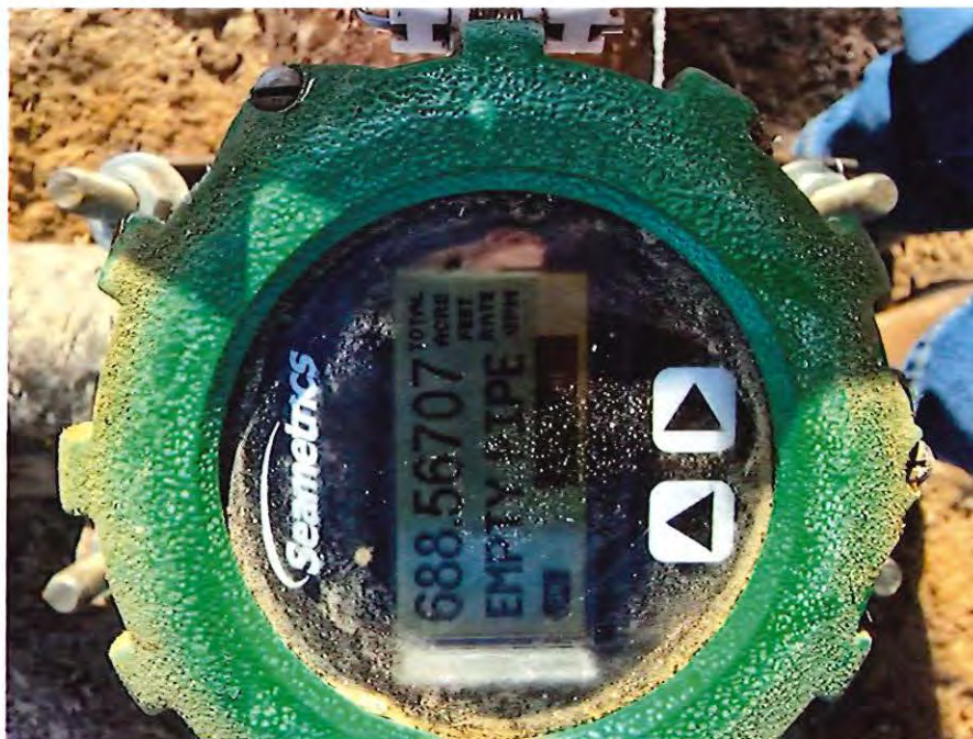
Flowmeter for Well #7
