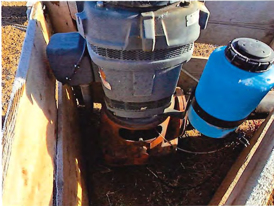
Pump and Motor Well #7
