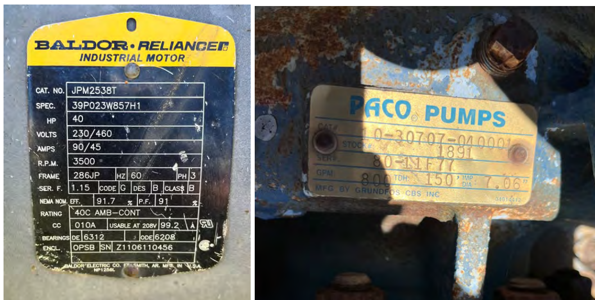
Figure 13. Photos of existing pump (photo credit NRCS 2024).
