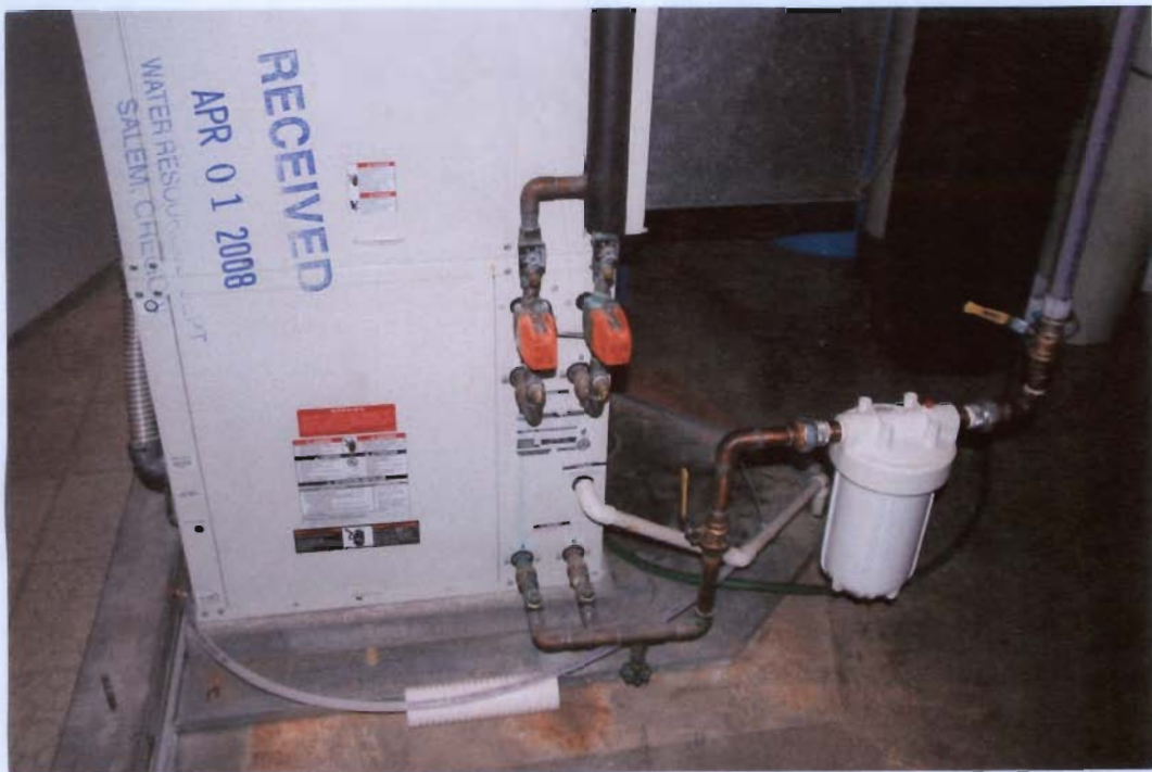
Left - Heat pump showing water filter and inlet. 2-26-2008
