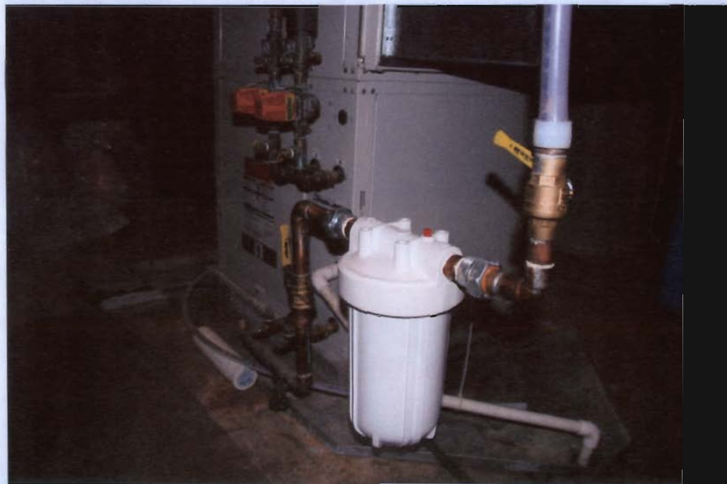
Left - Water piping from well source and filter w/ heat pump behind, 2-26-2008
