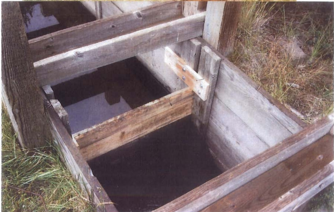
Main Diversion Box for Homesite 2007
