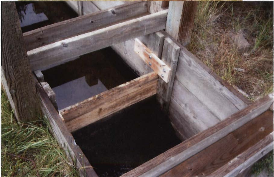
Main Diversion Box for Homestead 2007
