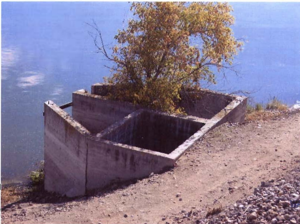
Existing Structure to be Remodeled and Used as Additional Point of Diversion
