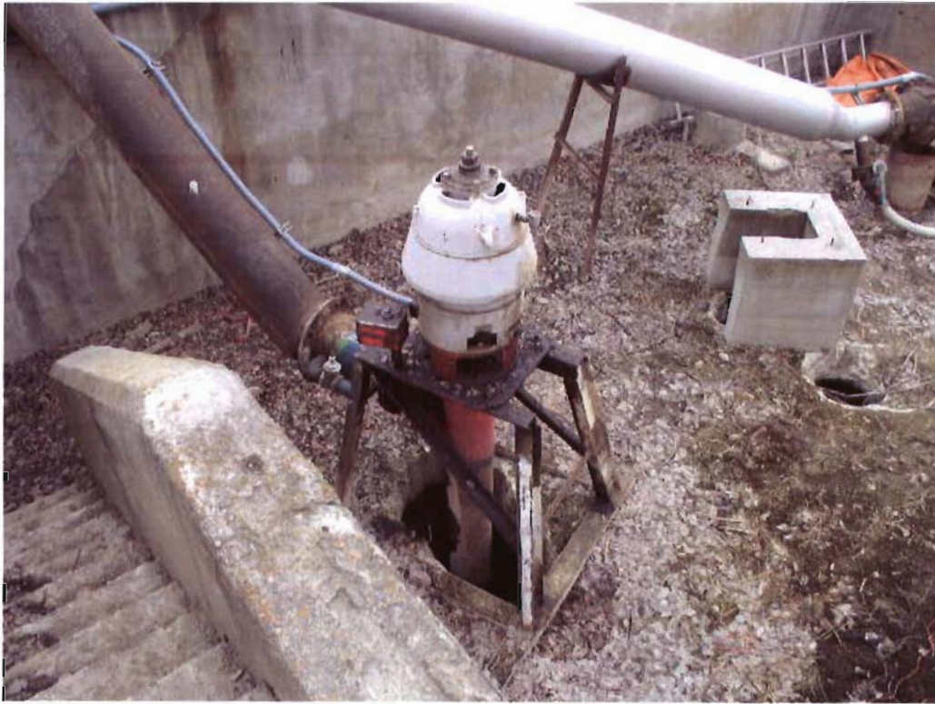
Existing Lift Pump at Existing Point of Diversion
