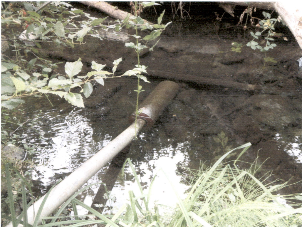
POD 1 Fish Screen in East Fork of Williams Creek
