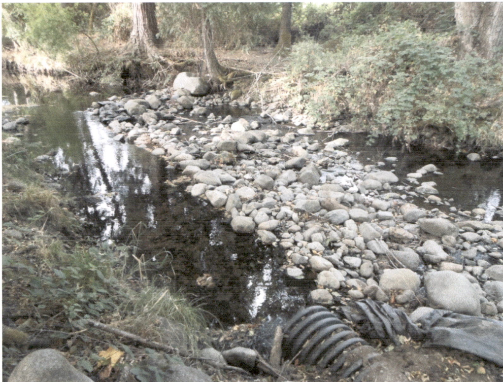
18" HDPE Pipe Inlet at "Spanish" POD
