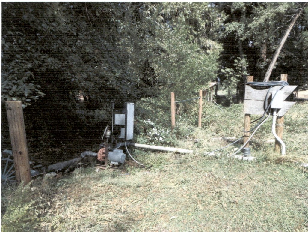
APOD Pump and Flow Meter
