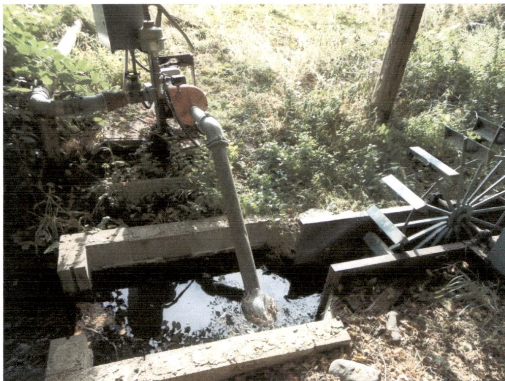
APOD Pump at Rotary Drum Screen
