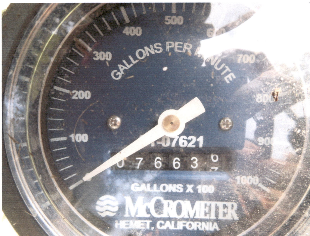
POD 1 Flow Meter
