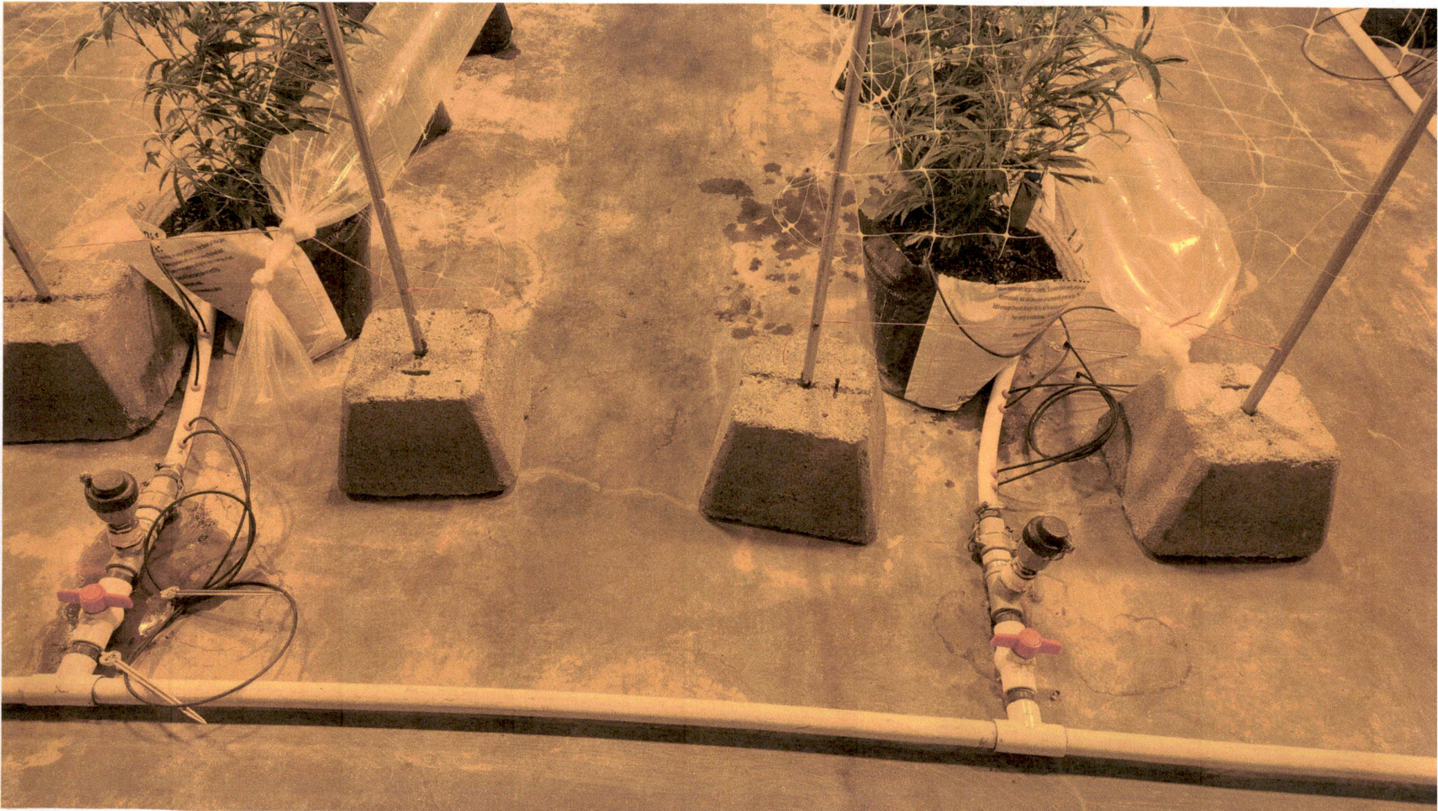
10-10-22 onsite Farrens COBBL 1 inch. supply lines to rows w/ emitters
