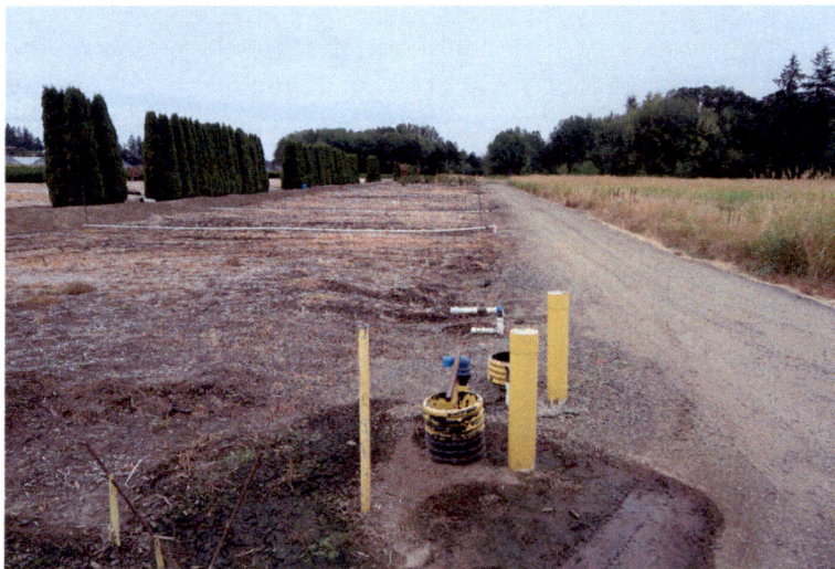
Irrigation set up in nursery with main valve in foreground.
