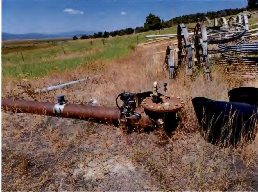
Well #3, Pressure Gauge, Control Valve & Flowmeter
