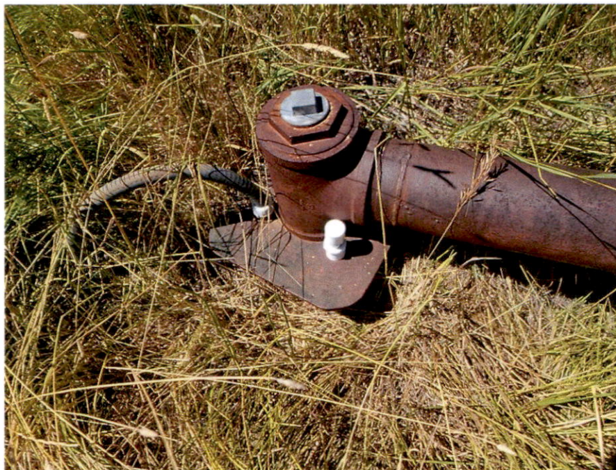
Well #2, Access Port
