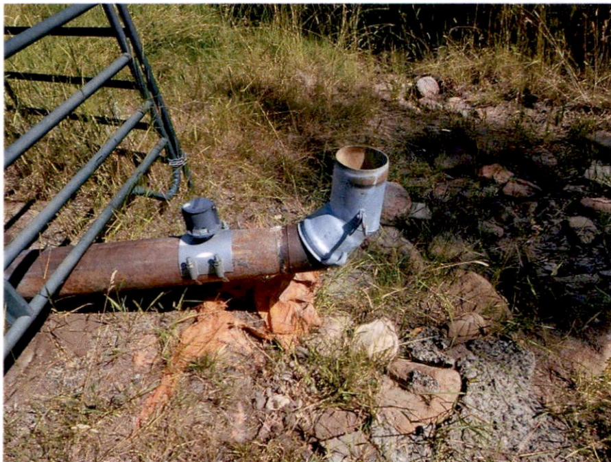
Well #1 Flowmeter & Discharge
