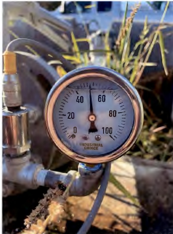
Photo of pressure gage showing operating pressure of the irrigation system. September 8, 2023. Photo provided by DIS Northwest, Inc.
