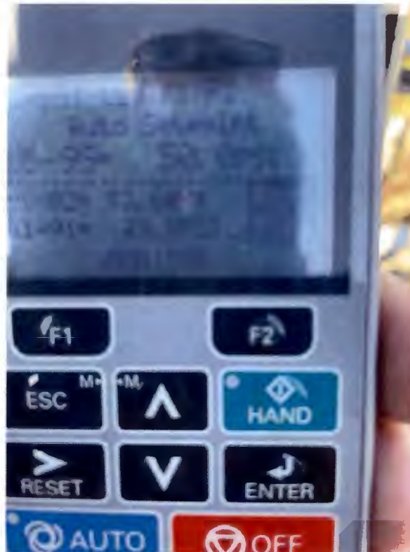
Photo of LED screen on the variable frequency drive. September 8, 2023. Photo provided by DIS Northwest, Inc.
