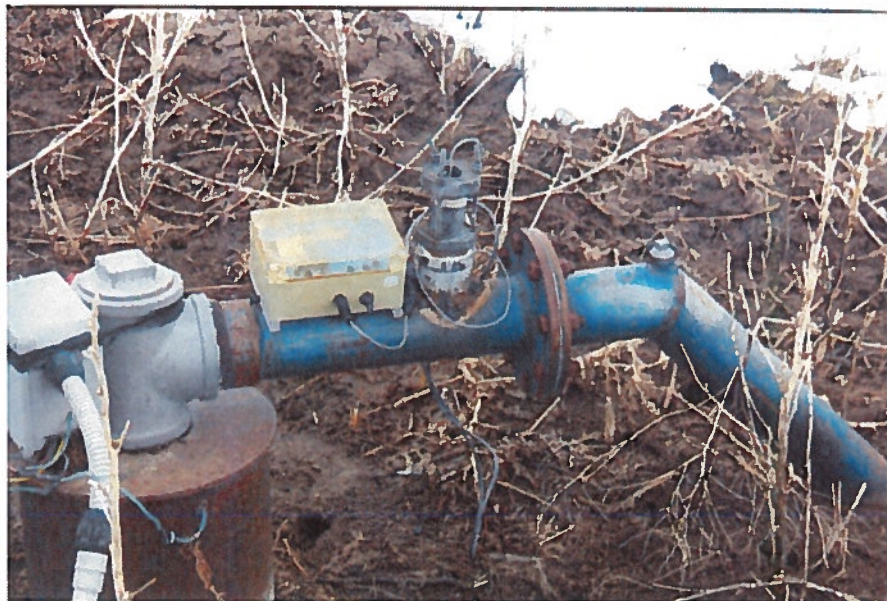
FLOWMETER AT WELL #2
