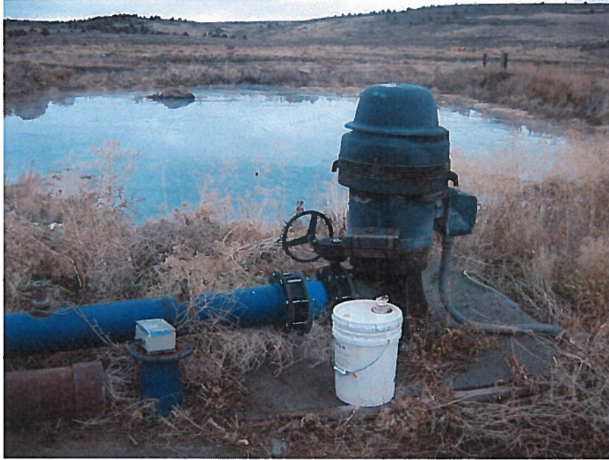
Pump at Pond for Pivots #1 and #2
