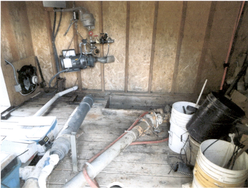
System: Inlet Pipe, Pump, Motor, Flow Meter
