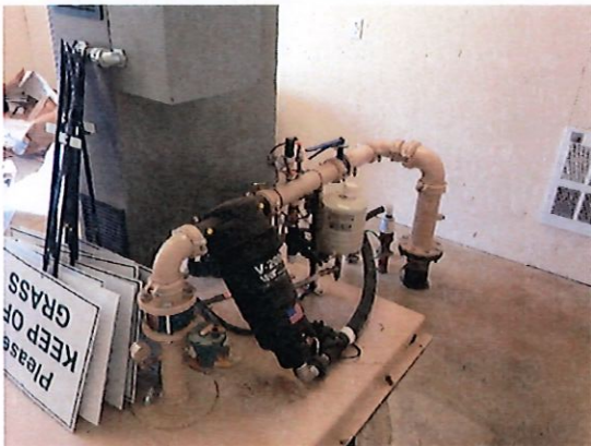
Irrigation pump station
