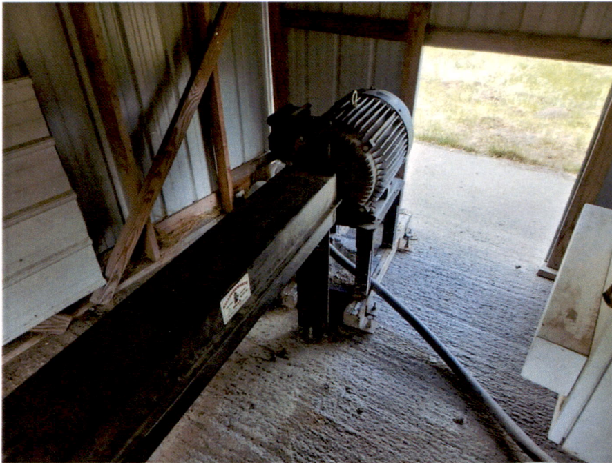
Well Pump Motor
