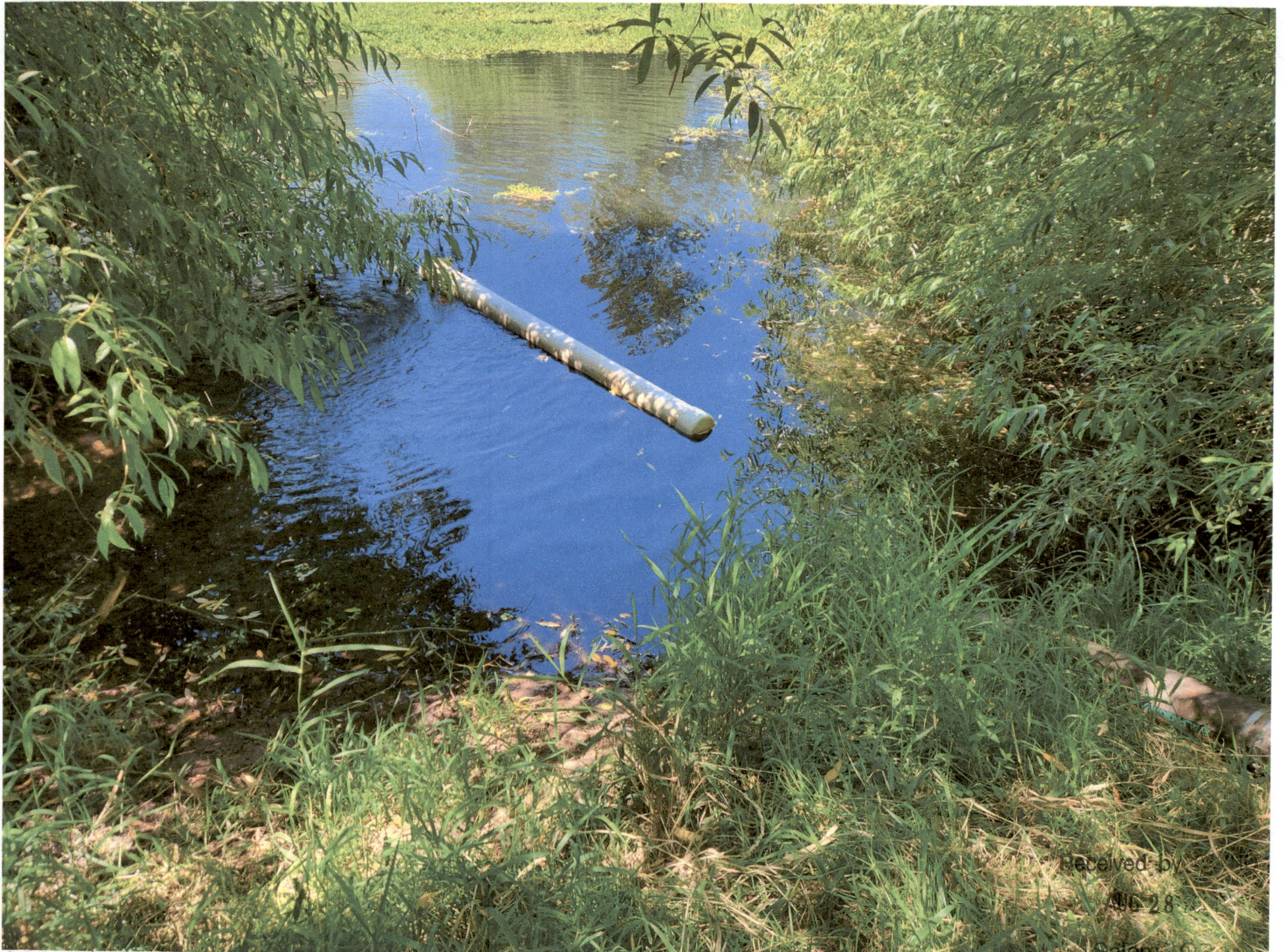
6-24-24 WEM Green Gold Ag COBU 30 HP Bulge Pump Suction line to fish screen
