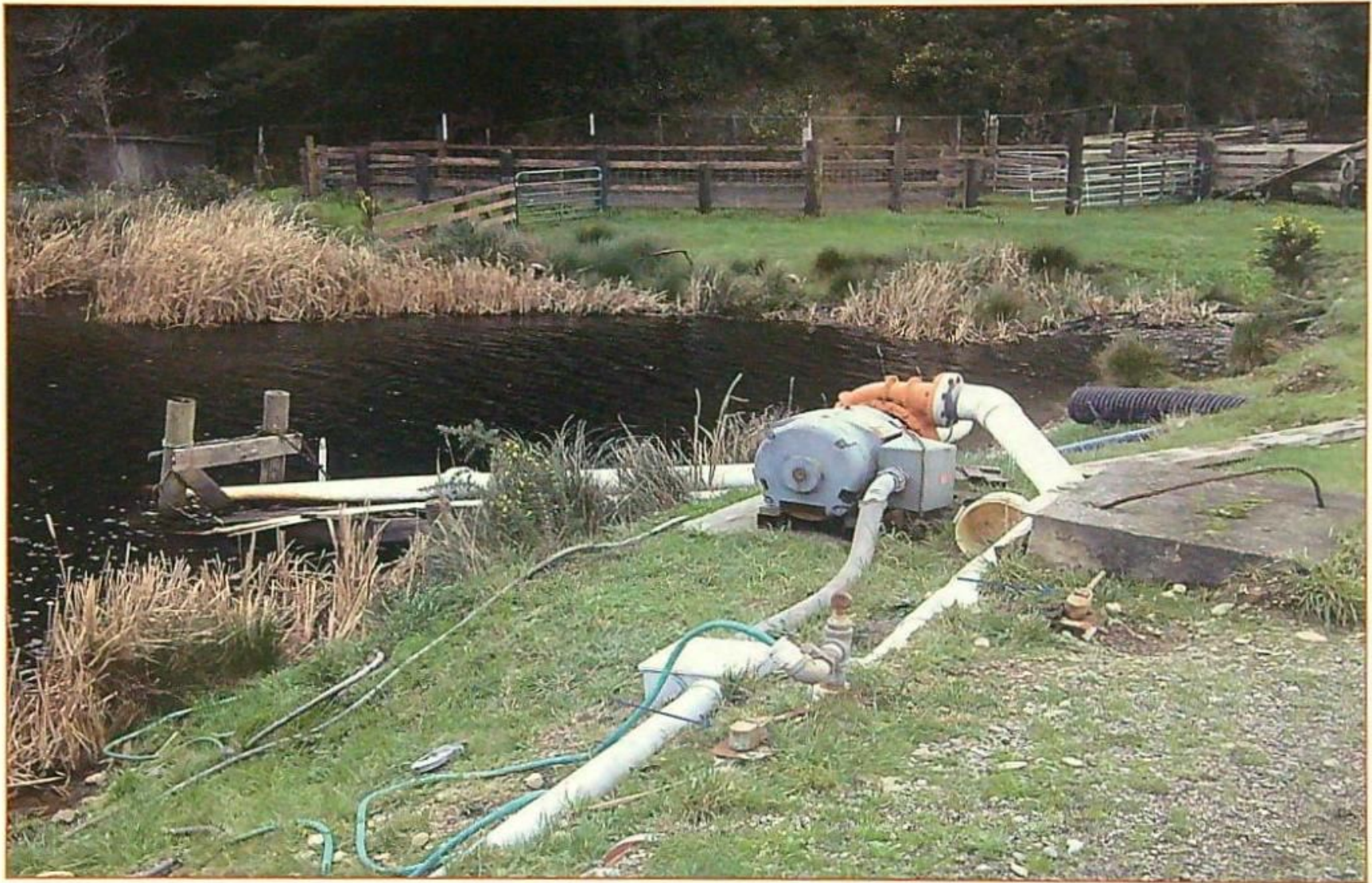
Knapp ranch irrigation system, looking WSW. Note valves in the foreground, the nearest controls water to the gravel wash plant and the other to the pastures.
