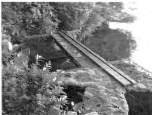
Outlet Control Structure on Woahink Lake
