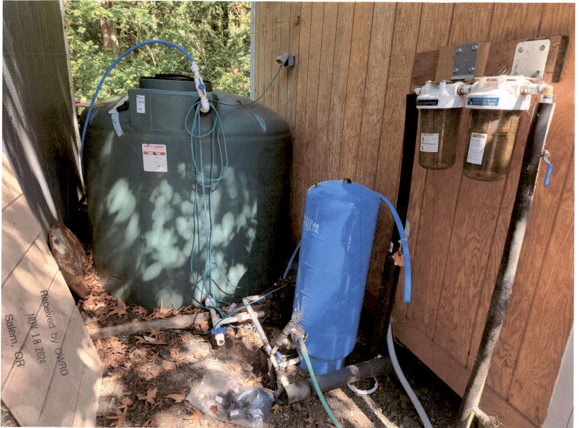
Brown COBU 9-13-2024 600 Gal. Storage Tank & Pressure Tank
