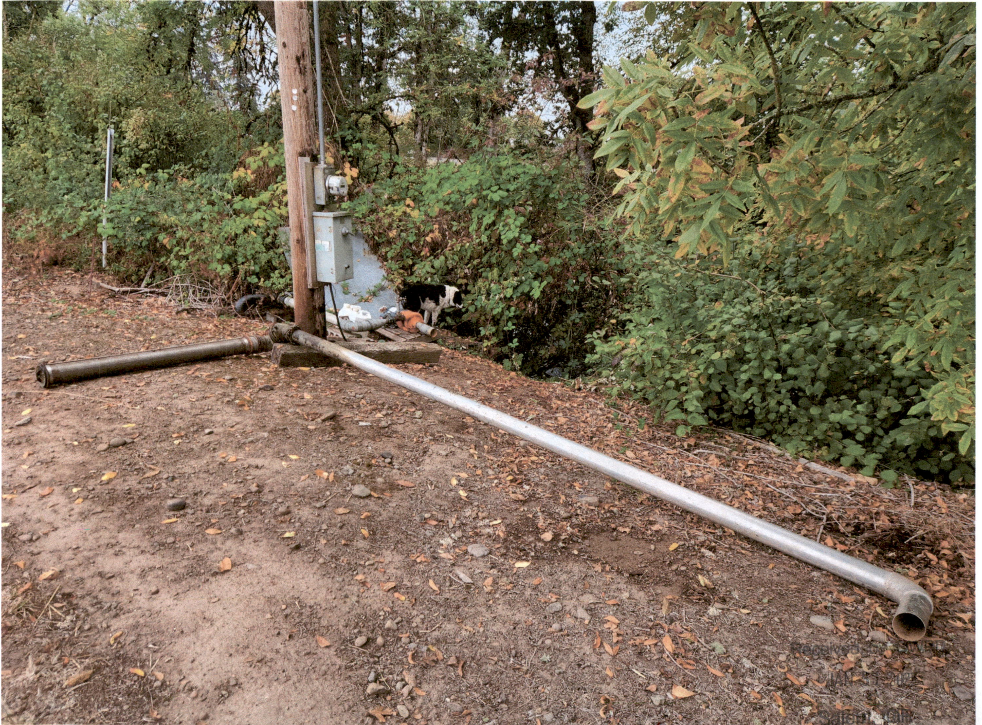
McGill 10-9-2024 Site Inspection — 7.5 HP pump, suction line & fish screen.
