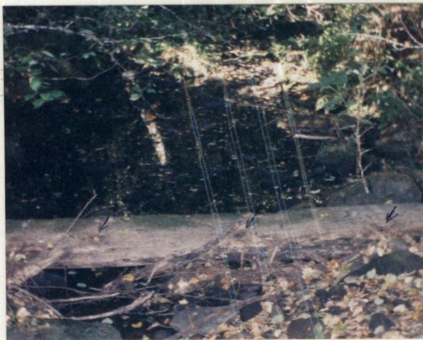
Rear sill of pre 1909 dam (looking downstream). Note flattened top from erosion by gravel and pin holes for beams on 3 foot centers. (see arrows)
