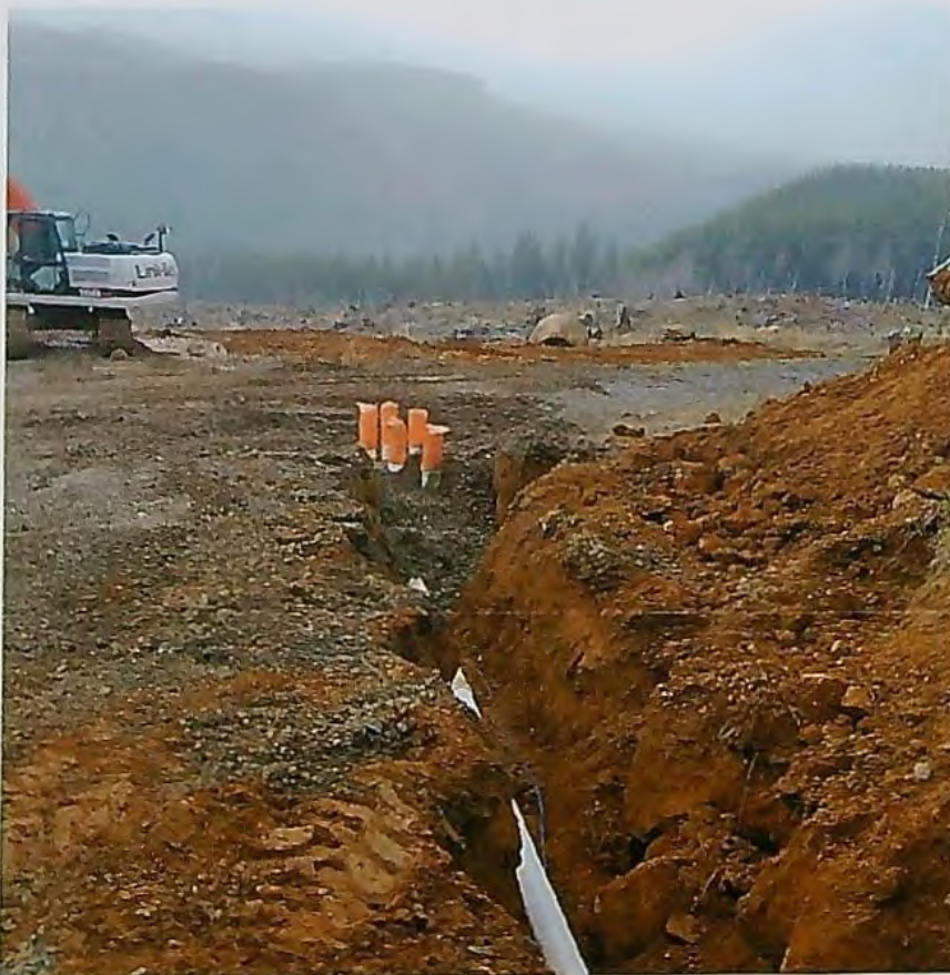
PHOTO 8 Intertie and overflow at connection to existing main transmission pipeline. 02-02-2018
