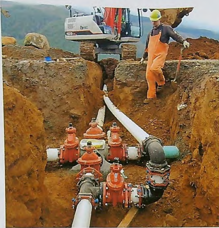
PHOTO 7 Intertie and overflow at connection to existing main transmission pipeline. 02-02-2018
