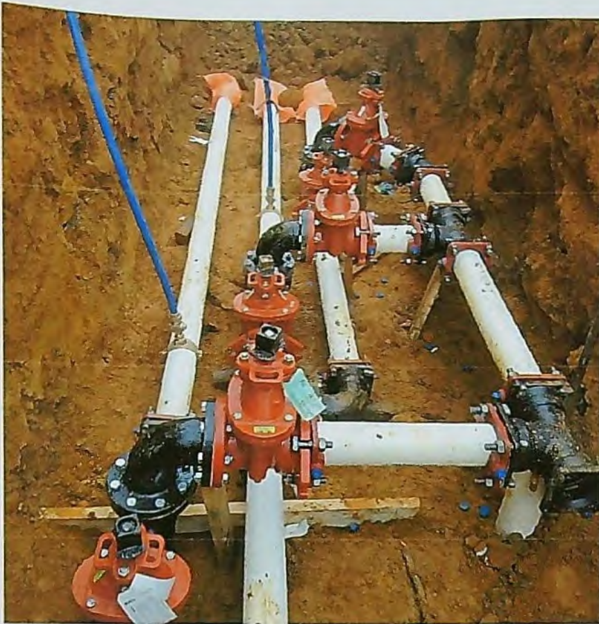
PHOTO 5 Sampling Station piping 01-08-2018
