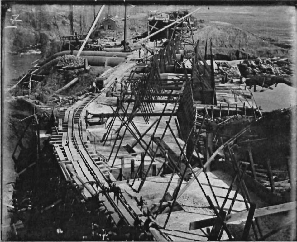
Cazadero - Penstock Intake at Forebay.
