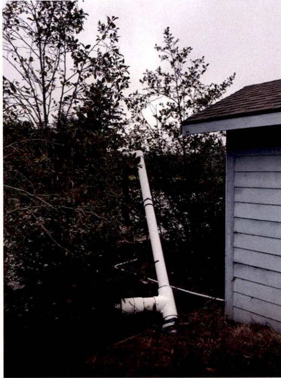
Reservoir 2, submersible pump plumbing alongside pump shed.
