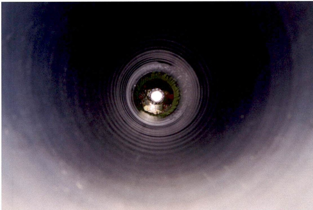
McCrometer totalizing meter at bottom of pipe. Pipe protects meter from high water and silt.
