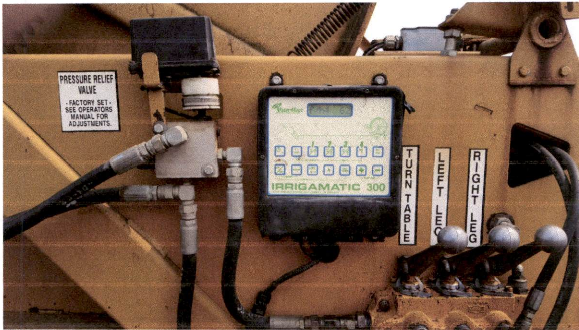
Photo 11: Irrigamatic control panel for big gun sprinkler.
