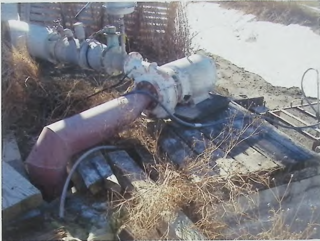
50hp pump connected to sand filter and C-4-C lateral.
