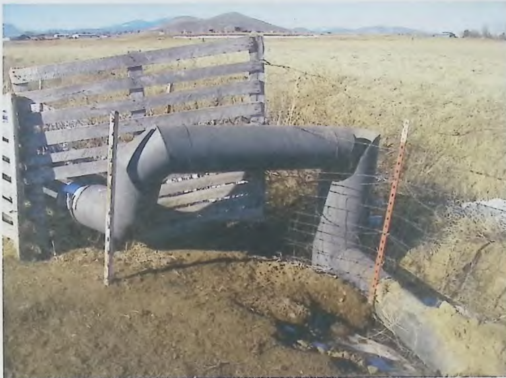
12" steel main and backflow preventer discharging into 18" steel pipe into ditch.
