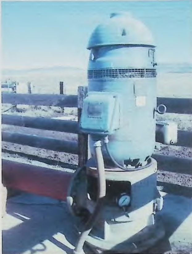
100hp motor on top of well casing with air line and pressure gauge.
