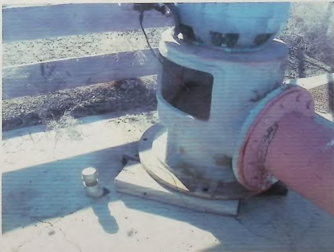
Well casing and 2" access port.
