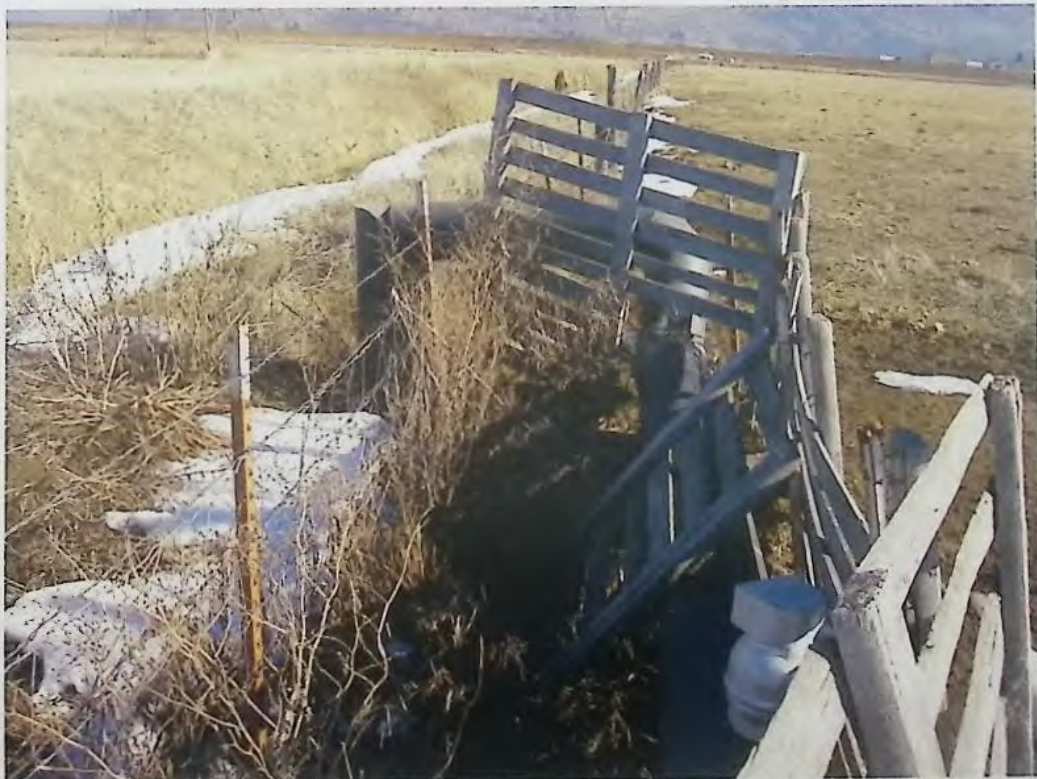
12" steel main at north end of property along ditch.
