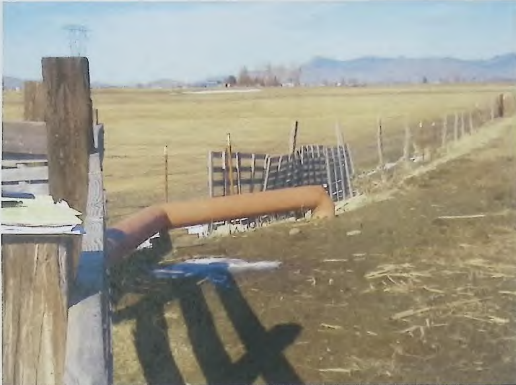
12" main as it goes underground and northerly along property line.
