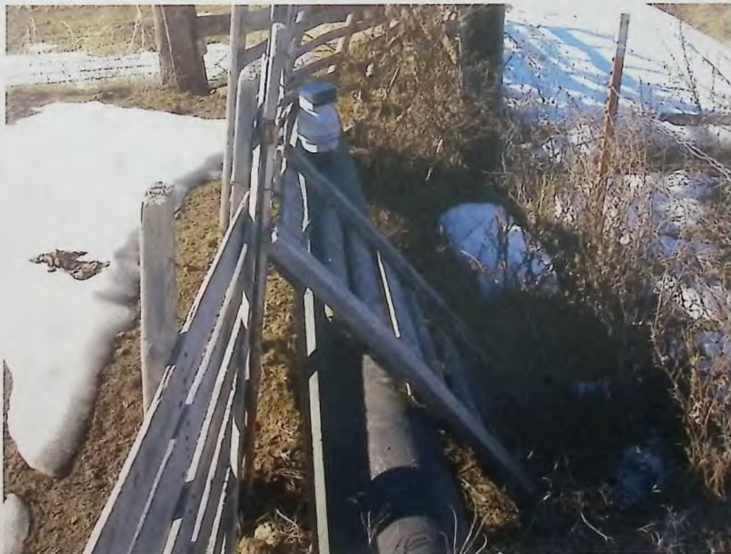
12" steel main resurfacing at north end of property showing air release valve.
