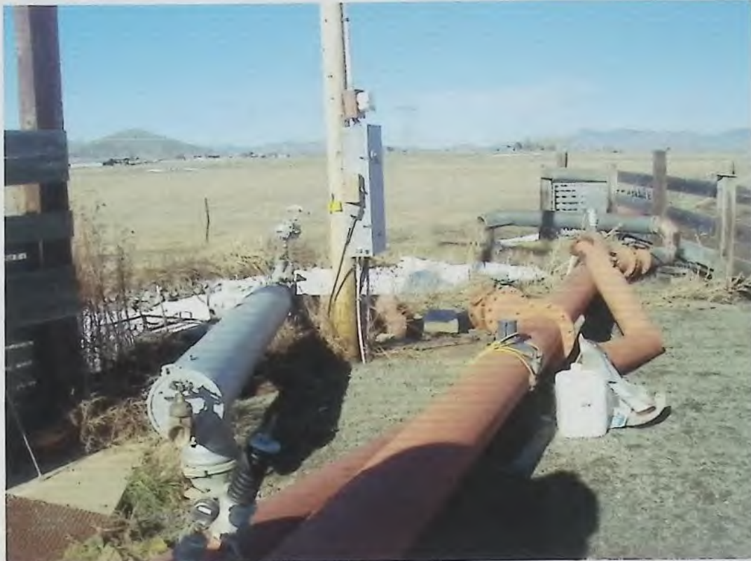
From pump looking north at filter and power
