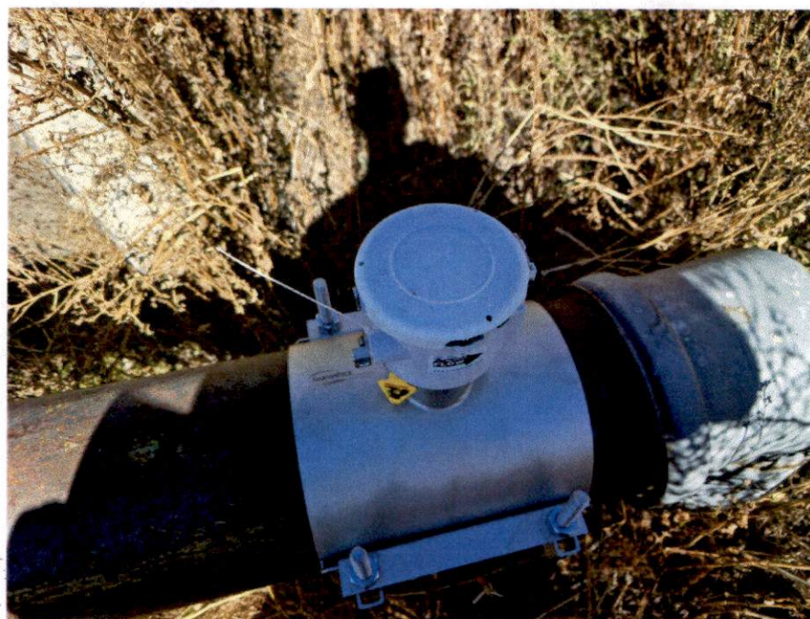
Hoefler Well Flowmeter
