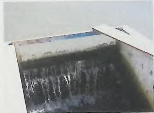
Thursday, April 04, 2002 Westbrook - 9s3w14 Ra-84703 Overflow pipe.
