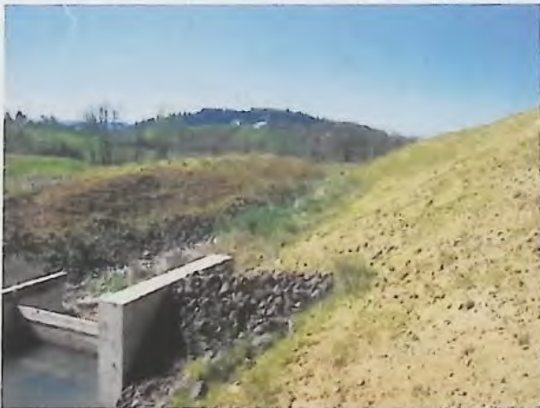
Thursday, April 04, 2002 Westbrook - 9s3w14 Ra-84703 Emergency spillway located on north end of dam.
