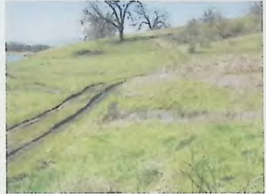
Thursday, April 04, 2002 Westbrook - 9s3w14 Ra-84703 Emergency spillway located on north end of dam. Spring area along north shore u.s. from emergency spillway.
