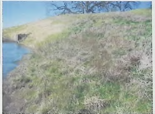
Thursday, April 04, 2002 Westbrook - 9s3w14 Ra-84703 Emergency spillway located on north end of dam. Spring area and slump.
