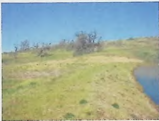
Thursday, April 04, 2002 Westbrook - 9s3w14 Ra-84703 Top of dam looking north. 6 of 6 panoramic shoots
