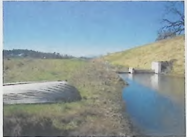
Thursday, April 04, 2002 Westbrook - 9s3w14 Ra-84703 Emergency spillway located on north end of dam.
