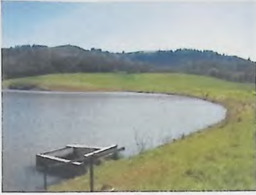
Thursday, April 04, 2002 Westbrook - 9s3w14 Ra-84703 Top of dam looking south. 1 of 6 panoramic shoots
