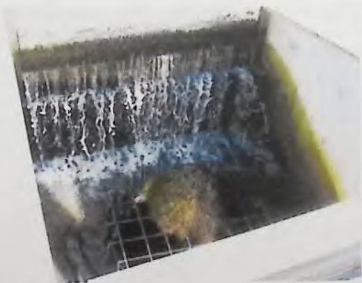
Thursday, April 04, 2002 Westbrook - 9s3w14 Ra-84703 Overflow pipe.
