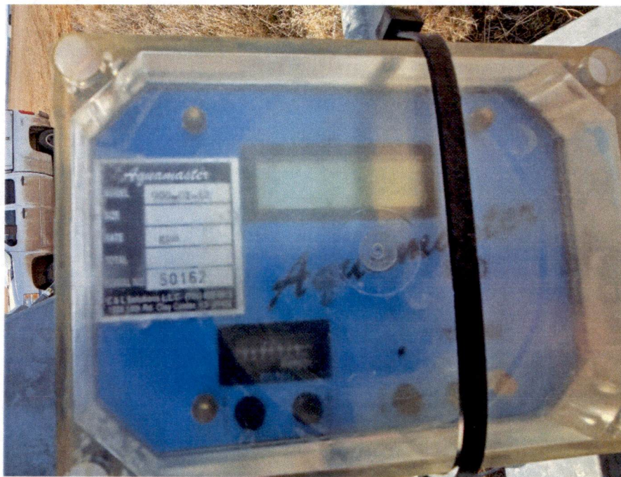
Well #8 Flowmeter Panel
