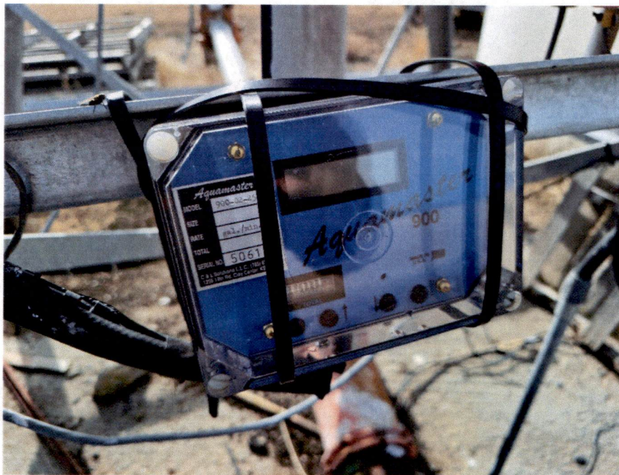
Well #9 Flowmeter Panel
