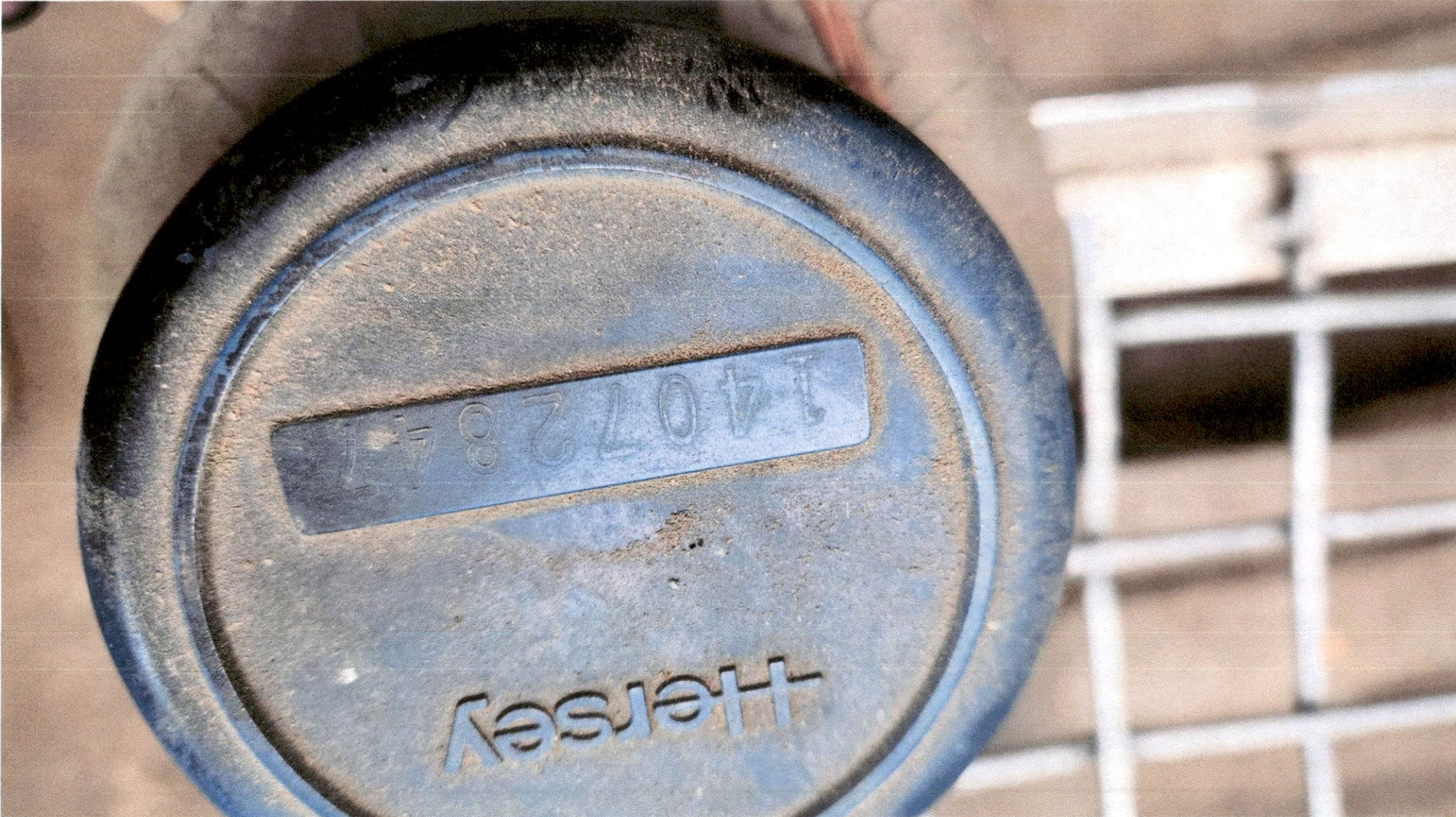
Dinsdale COBU 1 HP Flood Pump Flow Meter S/N
