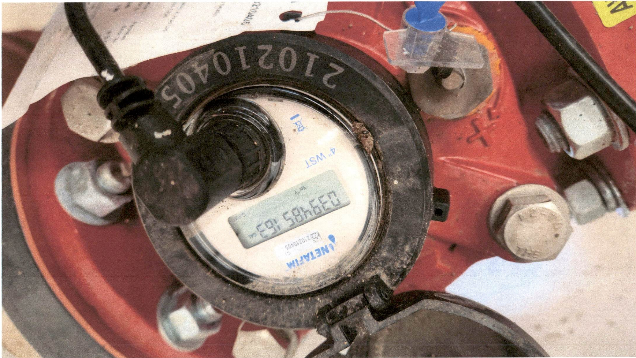
Perrott COBU Site Inspection 2-20-2025 Flow Meter
