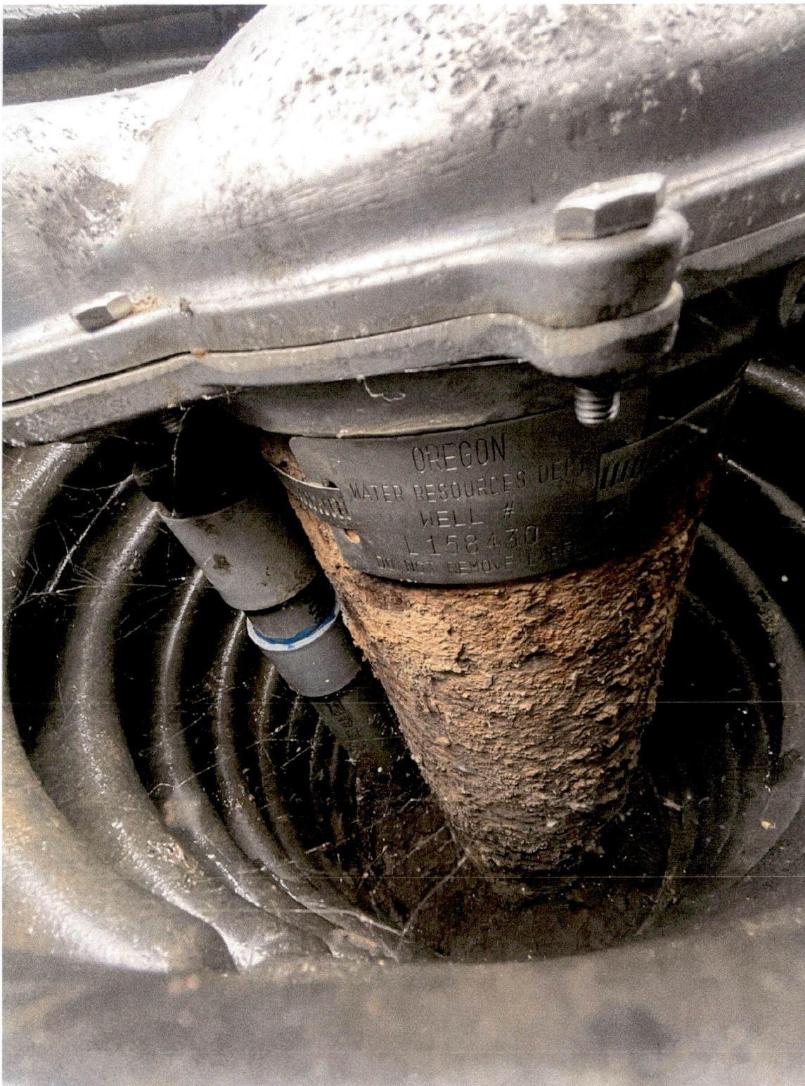
Photo: 02-20-2026 Well MARI 16968, L-158430 Tag installed September 3, 2025
