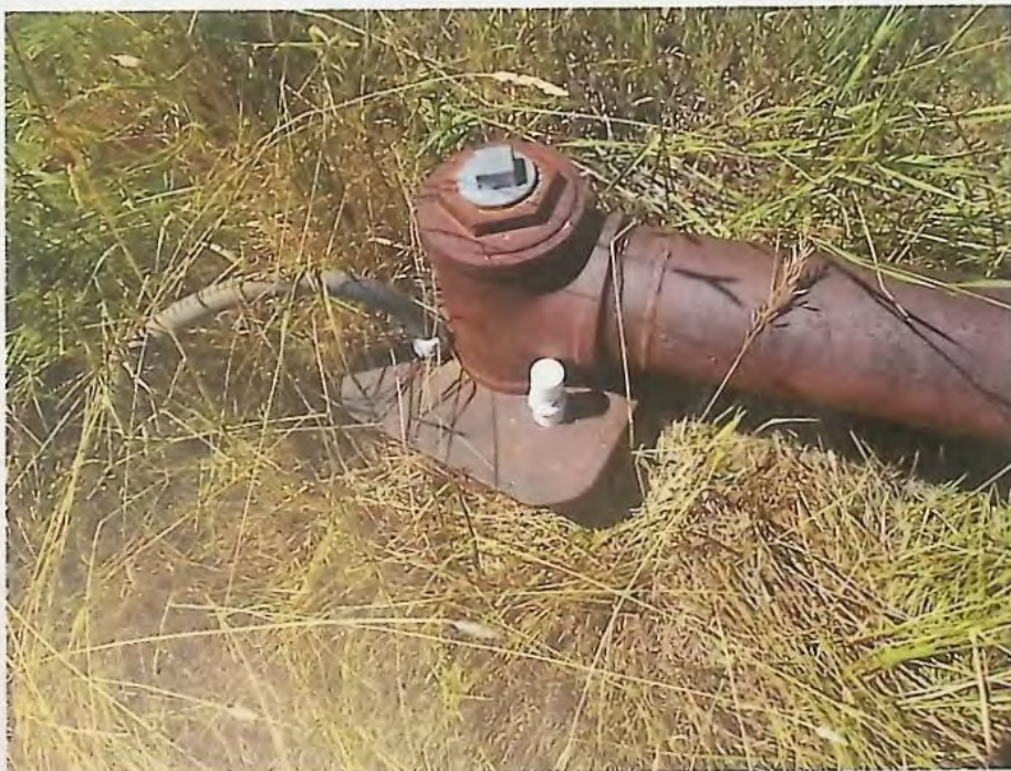
Well #2, Access Port
