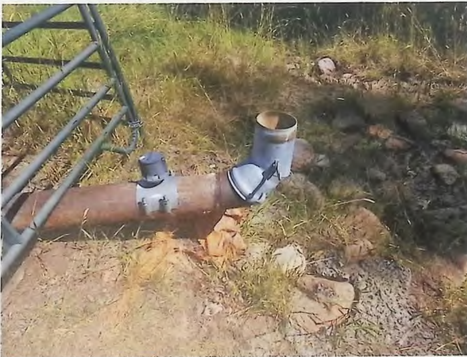
Well #1 Flowmeter & Discharge
