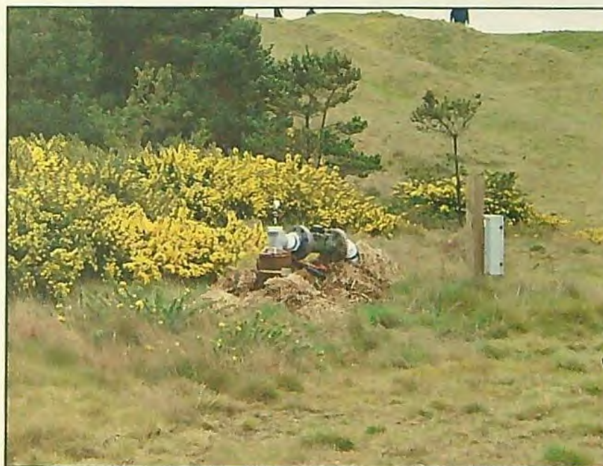
Photograph of Well L34008. Note the flow meter installation. All Bandon Dunes wells are equipped with similar meters and are monitored on a minimum monthly basis.
