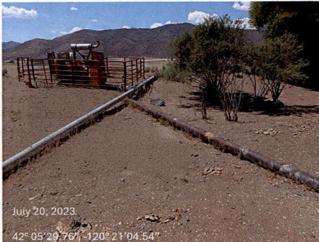
Figure 31. 100 kw Generator next to Turbine Pump and Well, looking west.
