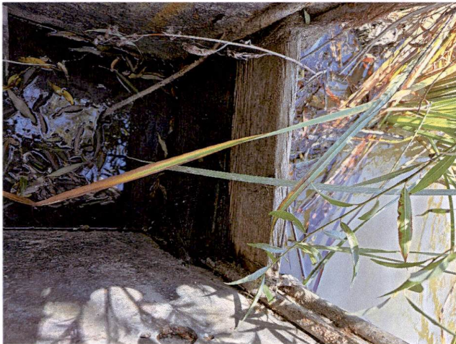
Typical Headgate structure
