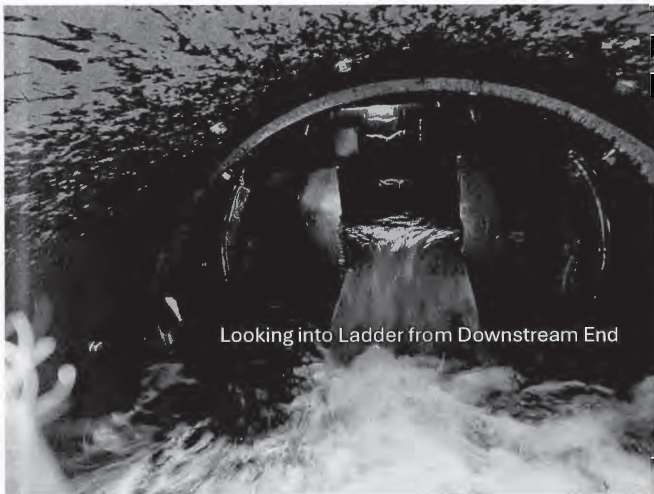
Figure 9. Simpson Creek "Amos" reservoir fishway outflow into the water collection gallery.
